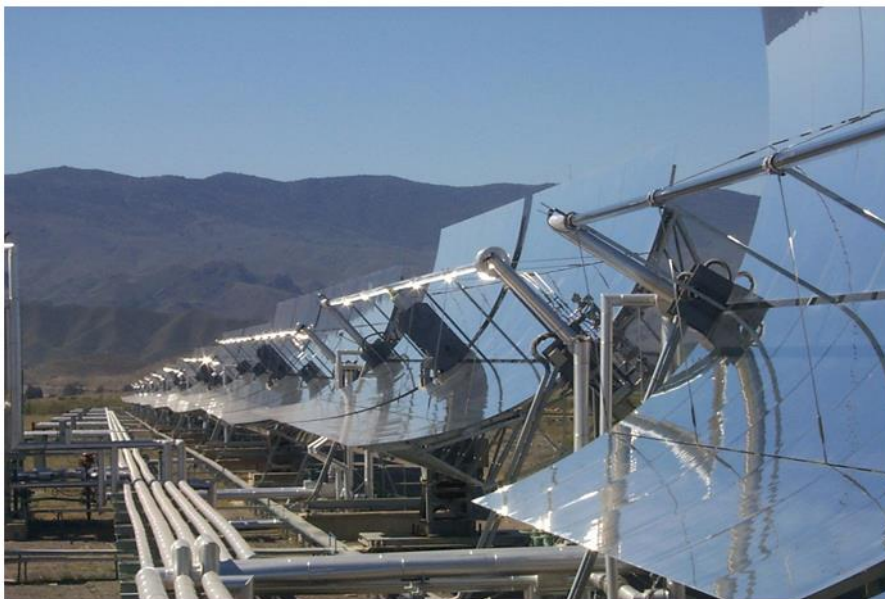
Figure 6: Parabolic trough power plant (DLR, 2005)
